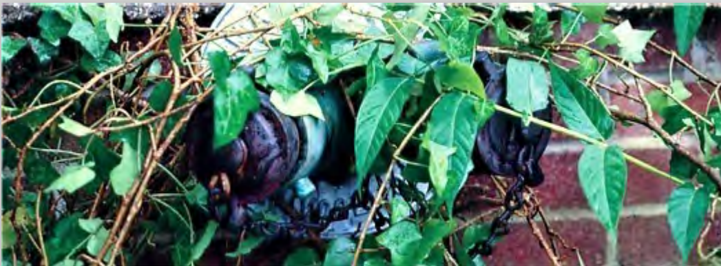
In the event of emergency, valuable time may be lost while the fire service searches for this connection hidden beneath overgrown vegetation.
