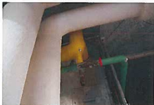
Photo 6 - Elbow Insulation Yellow
