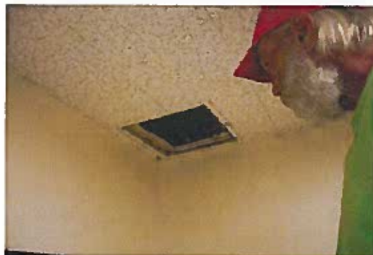
Photo 15 - Adhesive for Ceiling Tile
