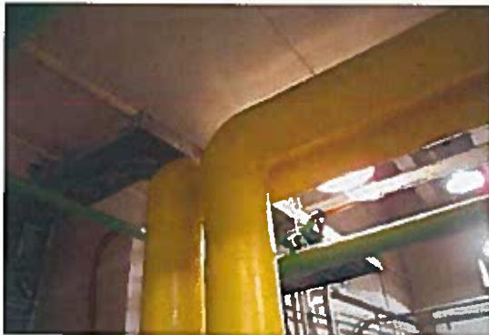
Photo 21 - Elbow Insulation Yellow
