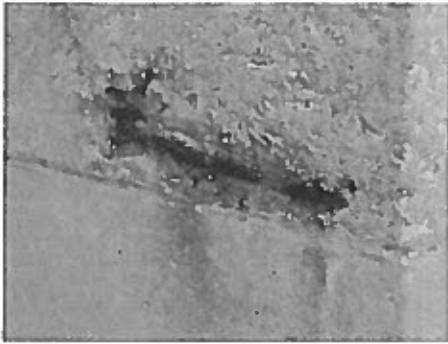
Shallow Concrete Cover
