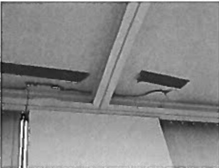
Spalls Within Adjacent Spandrel Beam
