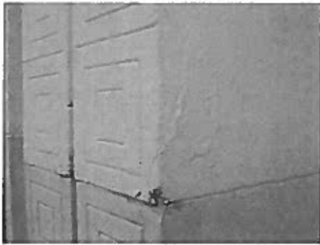
Existing Concrete Patches
