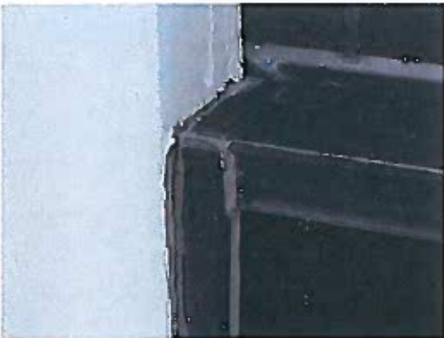
Failed Sealant Joints At Balcony Flashing
