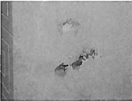
Corrosion Induced Spalls
