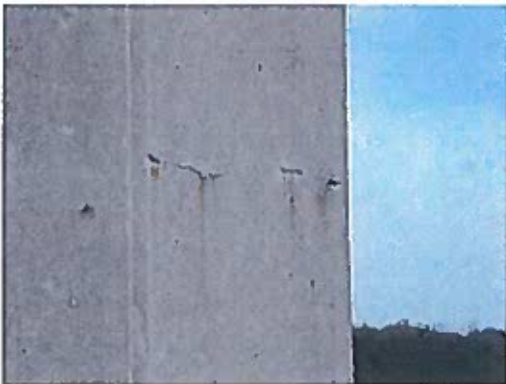
Shallow Concrete Cover.
