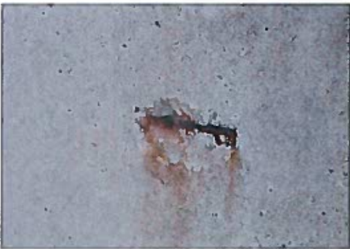
Corrosion Induced Spalls
