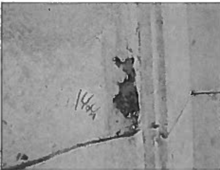
Spalls of Poor Concrete Consolidation.
