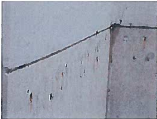
Spalls at Post-Tensioning Anchors
