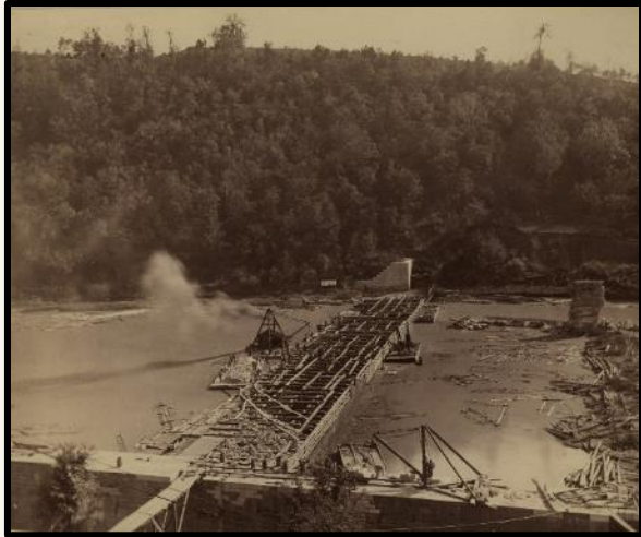
Lock No. 5 under construction near Tyrone circa 1885. Courtesy of the National Archives.
