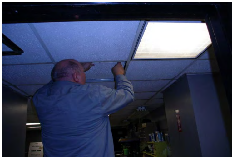
Sample 95 Ceiling tile Ground floor
