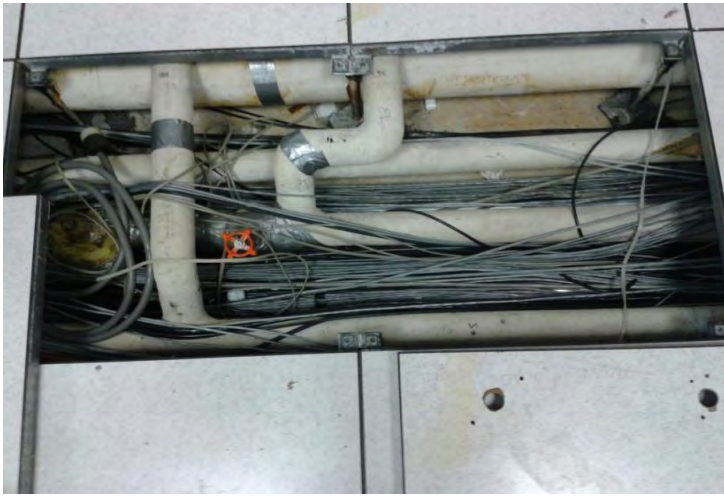
Photo 1 Pipes under floor tile Fourteenth Floor
