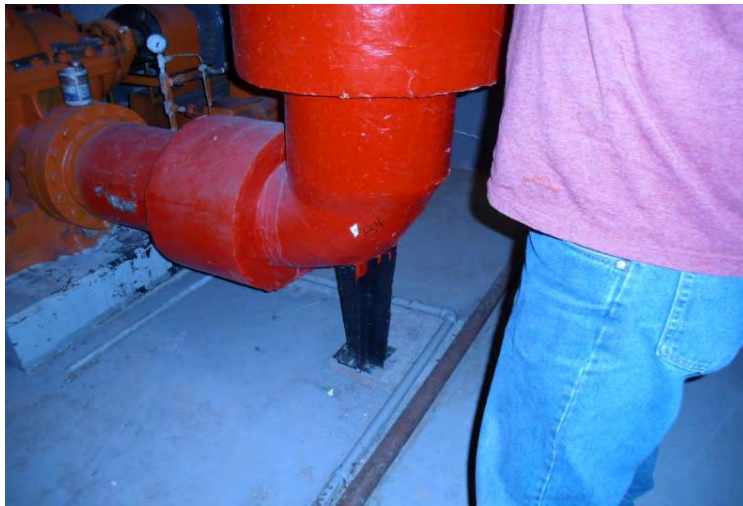
Sample 84 Elbow Mechanical Room
