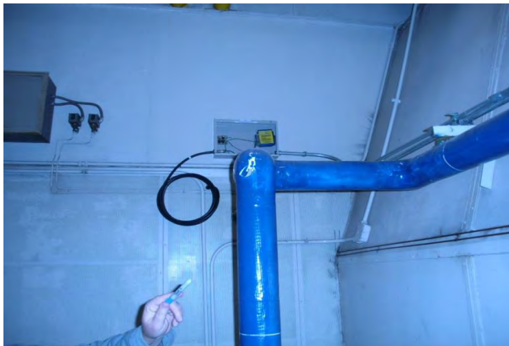
Sample 13 Elbow insulation Floor 13A
