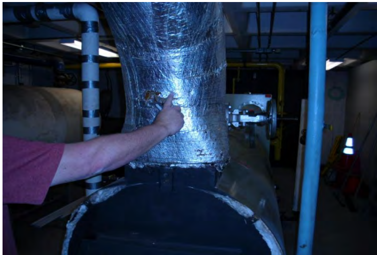
Sample 76 Pipe wrap tank Boiler Room
