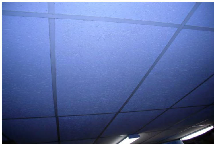
Sample 94 Ceiling tile Ground floor
