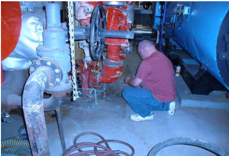
Sample 72 Elbow Boiler Room
