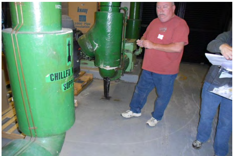
Sample 81 Valve wrap Mechanical Room
