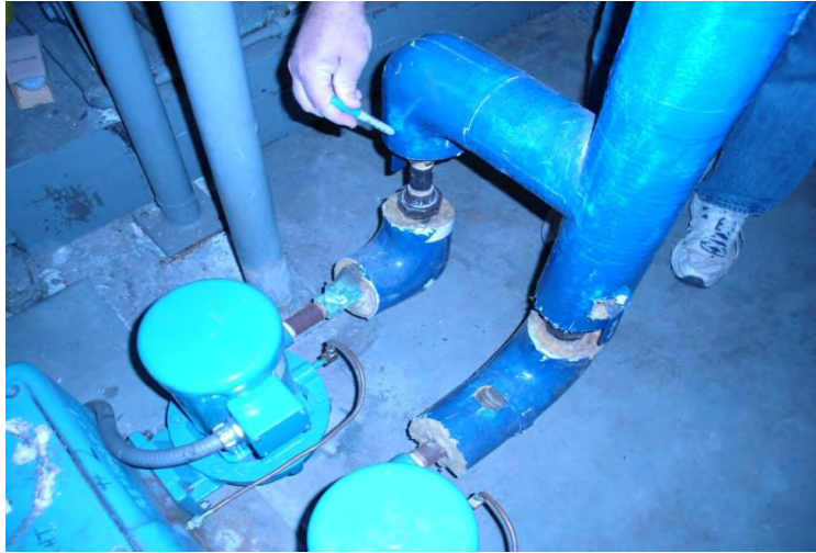
Sample 11 Elbow pipe insulation Floor 13A
