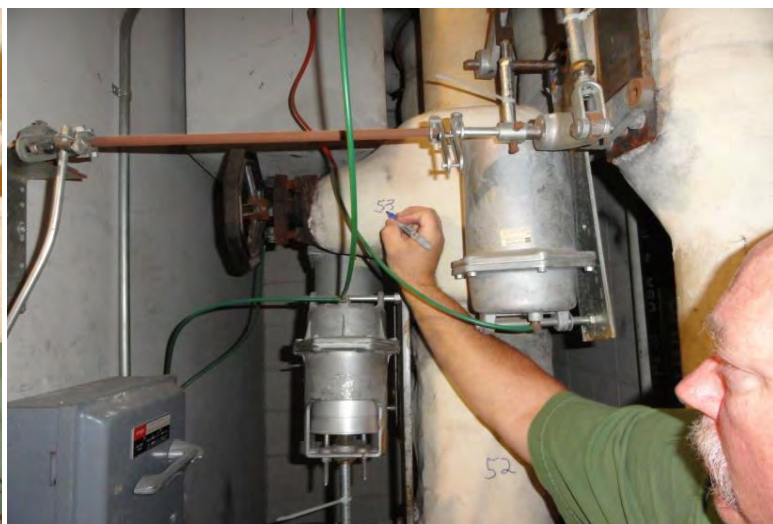
Sample 53 Pipe Wrap on valve Floor 13B
