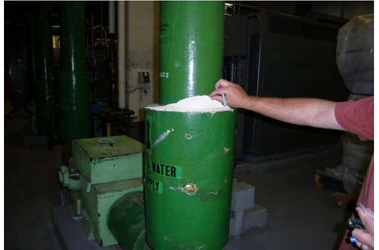
Sample 79 Valve junction Mechanical Room
