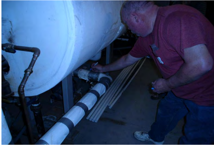
Sample 74 Pipe wrap tank Boiler Room
