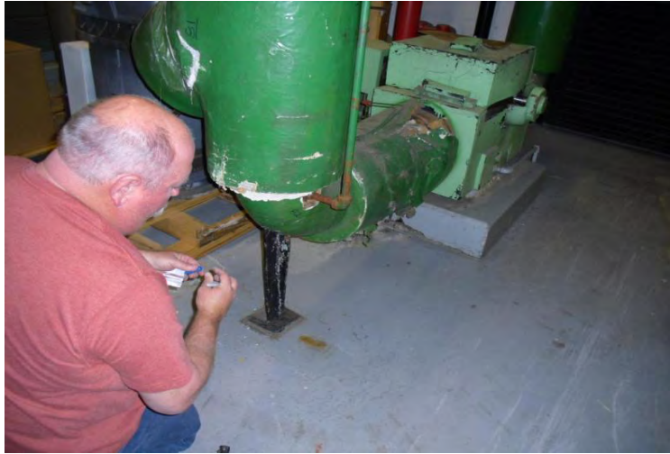
Sample 82 Elbow Mechanical Room
