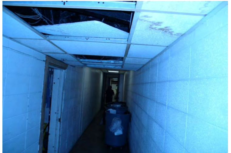
Sample 87 Ceiling tile Ground floor
