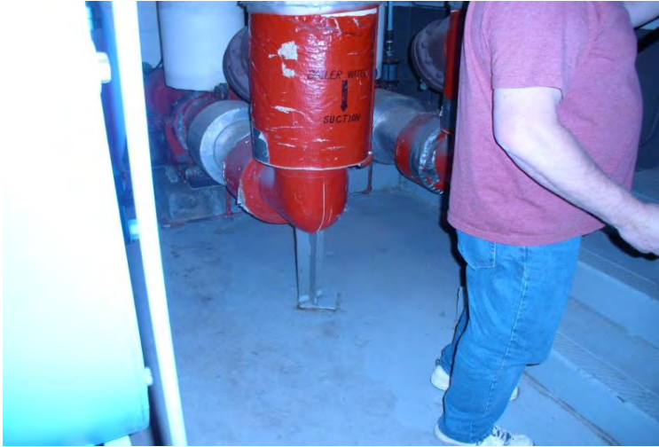
Sample 70 Elbow Boiler Room
