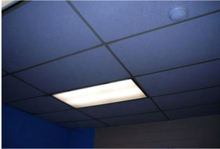
Sample 86 Ceiling tile Ground floor
