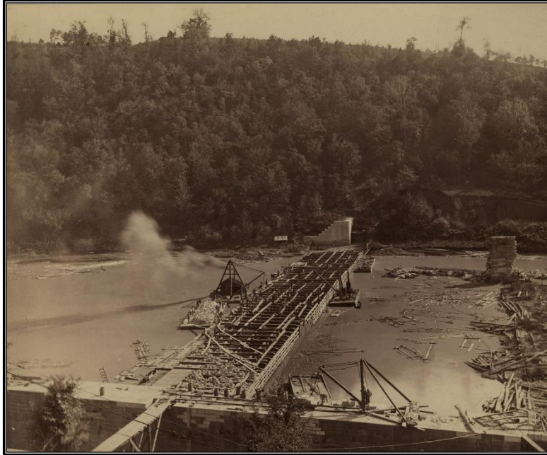
Image 7. Construction of the timbercrib dam at Lock and Dam No. 5 circa 1885. From the Records of the Office of the Chief of Engineers, 1789–1999 housed at the National Archives, online at the National Archives Catalog, https://catalog.archives.gov/ .
