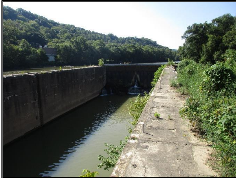
Image 7. View of lock chamber and lower gates looking upriver, circa 2016. Courtesy of Cultural Resource Analysts, Inc.
